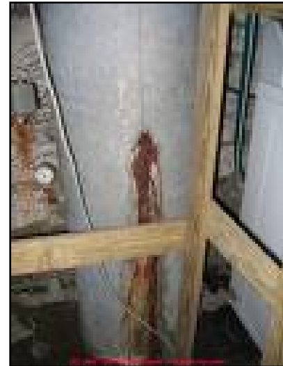
Rust streaks may indicate leakage
